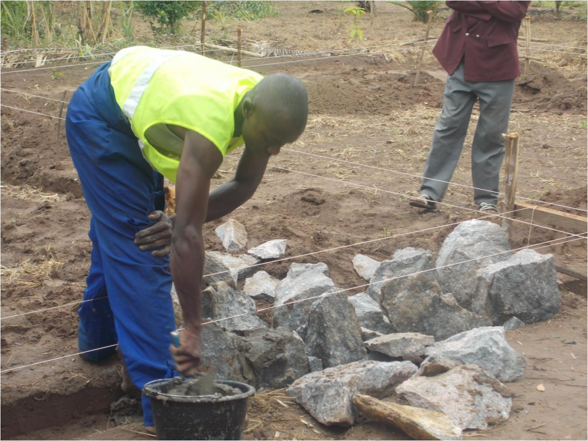
Building of the foundation in nature stones. The foundation was completed by 8 February.
