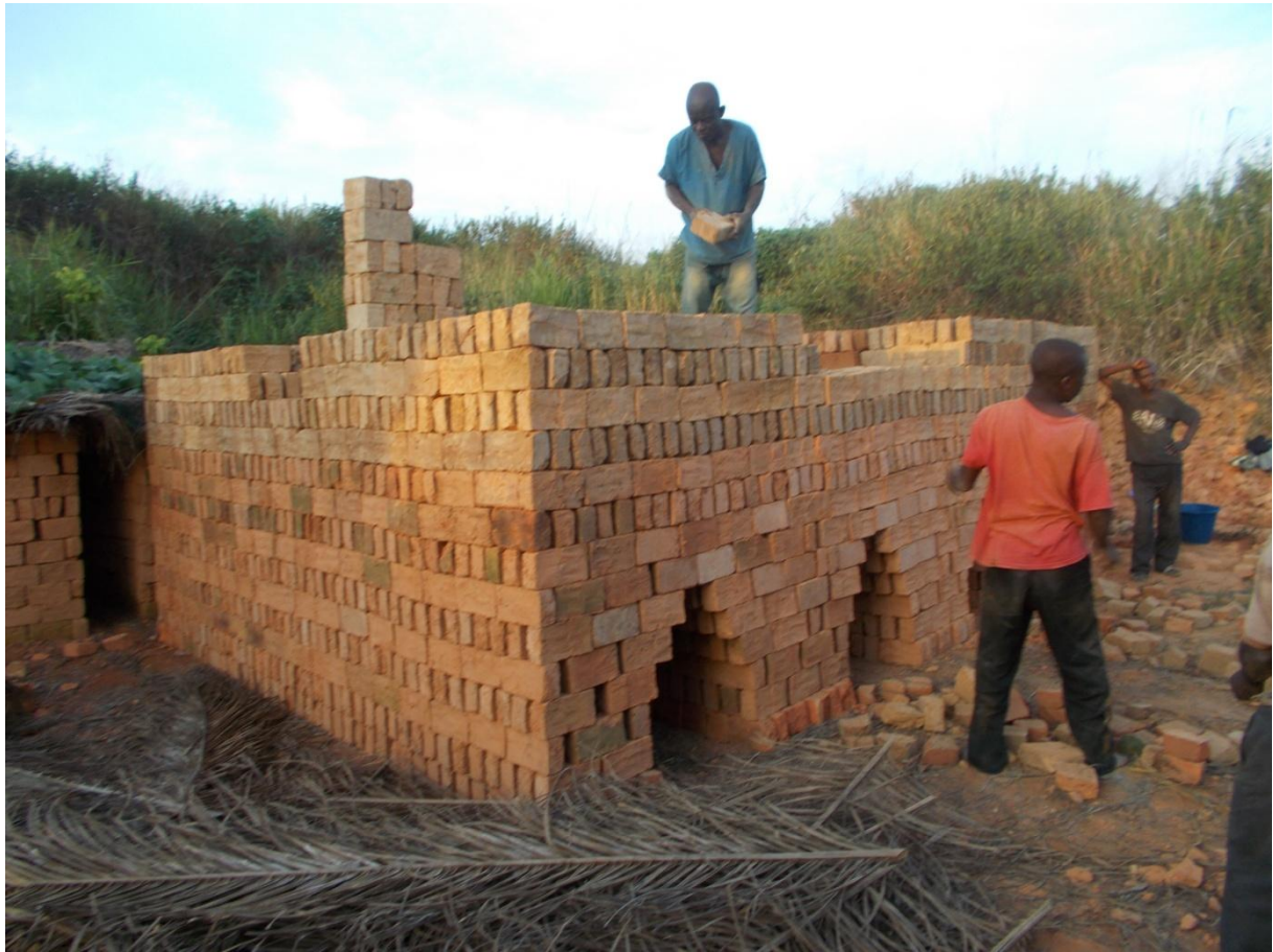
Construction of one of the 3 ovens made of compacted mud bricks to be burned. 24 to 36 hours, under constant supervision. The duration depends on the dimensions of the oven.
